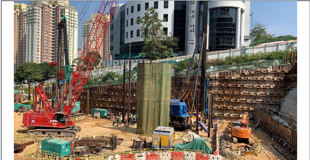
Hoisting of noise barrier during piling 打樁過程中隔音屏障的吊裝 打桩过程中隔音屏障的吊裝
